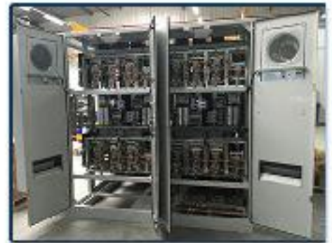
BGR - Control Panels, Rectifiers
